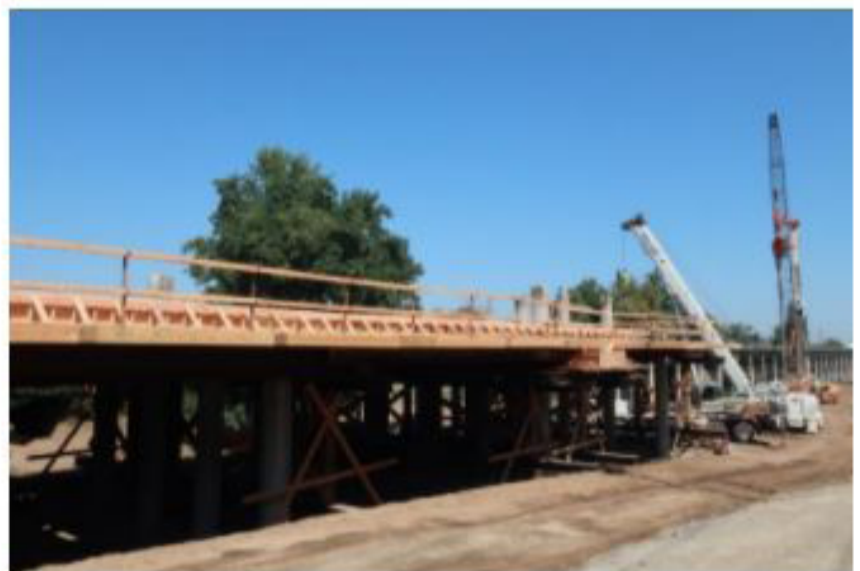
Falsework and forming for the bridge deck at the Southern end on the Stanislaus River.
