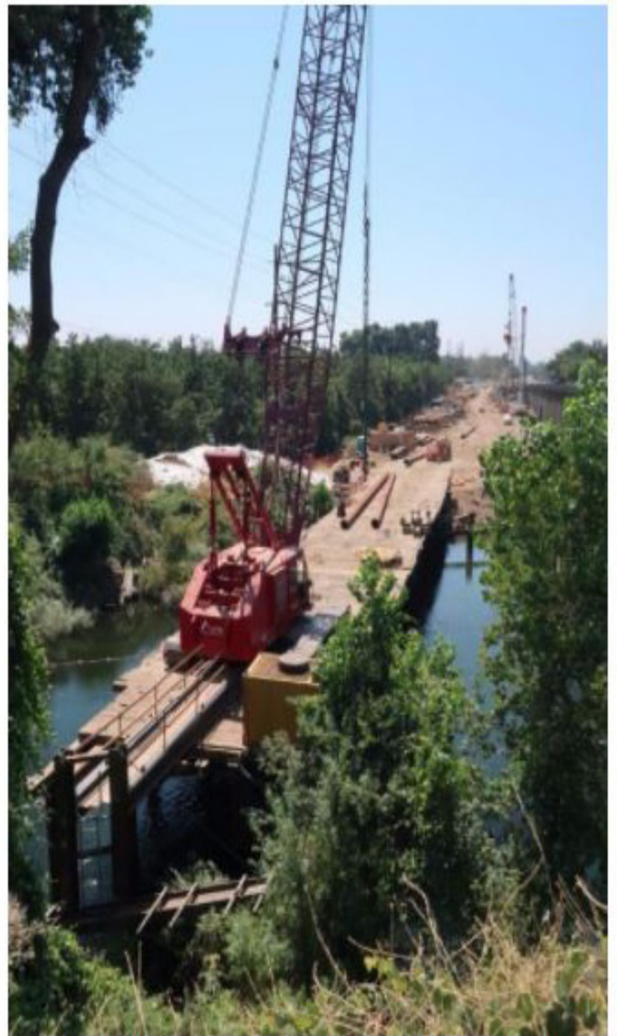
Temporary trestle over the Stanislaus River to allow crews access for construction equipment.
