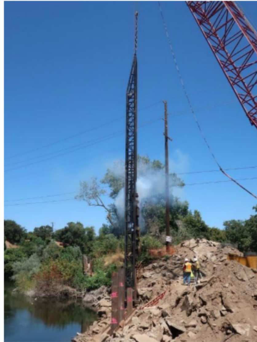
Construction crews driving steel piles for support of the temporary construction trestle
