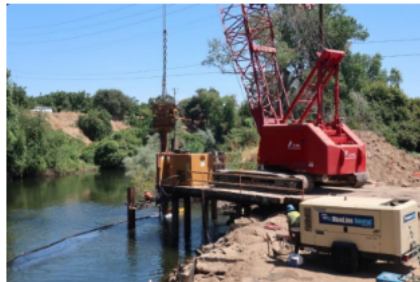
Construction of the temporary trestle to allow access to construct the bridge.
